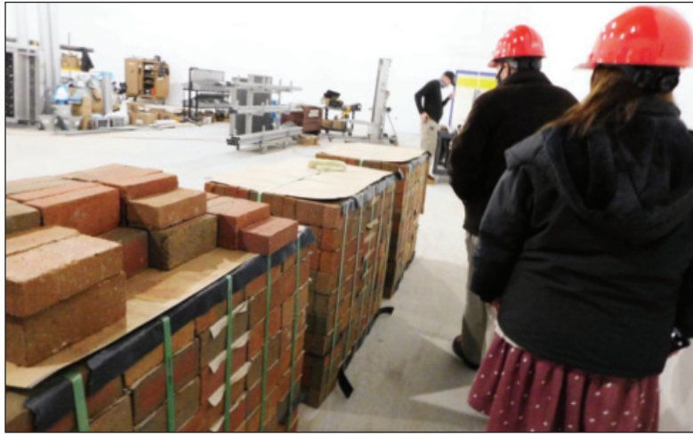
Bricks are temporarily stored in the new gymnasium to warm up prior to installation. (Cleaver photos by Dianne Alward-Biery)
